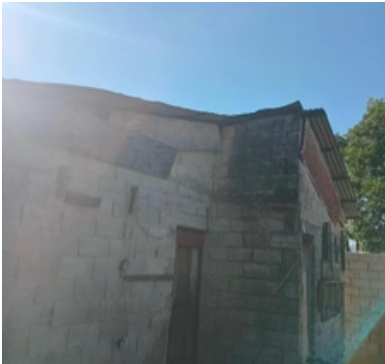
Deacon Simpson's Damaged Home
